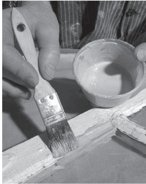
Figure 5 Liquid putty is brushed into small cracks in the front putty. This is a simple measure to delay ageing.
