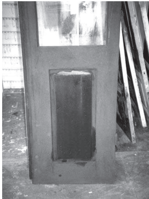
Figure 3 Maintenance of an old door, after nine years, with boiled linseed oil or linseed-oil wax.
